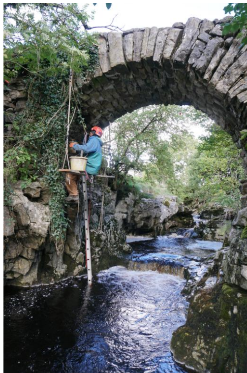
Fig. 16.2 Thorns Gill footbridge in 2018 undergoing structural repairs undertaken by Pete Roe, heritage builder (YDNPA HER)
