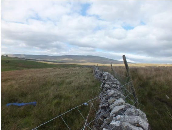
Fig. 9.26 Wall no. 15 runs off far into the distance heading westwards towards Ribblehead viaduct – with 100m tapes running down the wall side (Phil Carroll)
