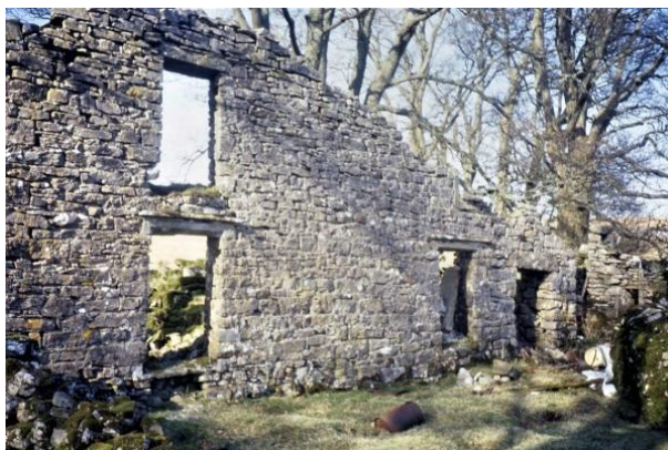
Fig. 10.9 Thorns 1, front elevation in 2003, prior to collapse (David Johnson)
