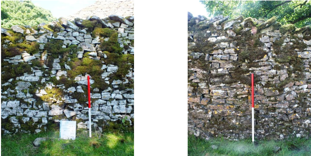
Fig. 9.27 The effects of weathering and plant growth on two sides of the same wall profile on Wall no. 29 (Phil Carroll)
