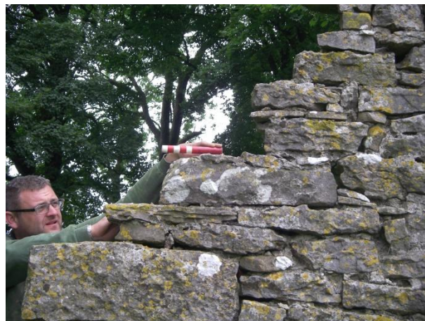
Fig. 15.4 The outer face of the reused fire window lintel, with Simon, one of the building team, holding the 200mm scale (David Johnson)
