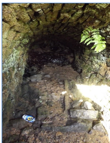
Figure: 33 The entrance to the Kinning Mine Level [GS6]. The tunnel entrance has collapsed further in.
