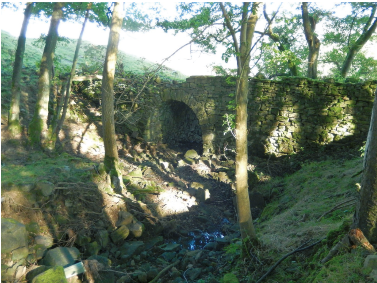
Image 22: Mill Field. Above the dam and mill pond. Juniper Gill exits Juniper Gill Plantation under this bridge.
